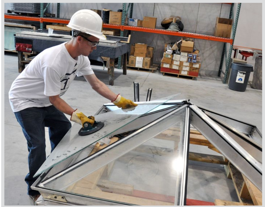
An apprentice at the Finishing Trades Institute of the Upper Midwest in Little Canada, Minn., demonstrates setting glass panels.
